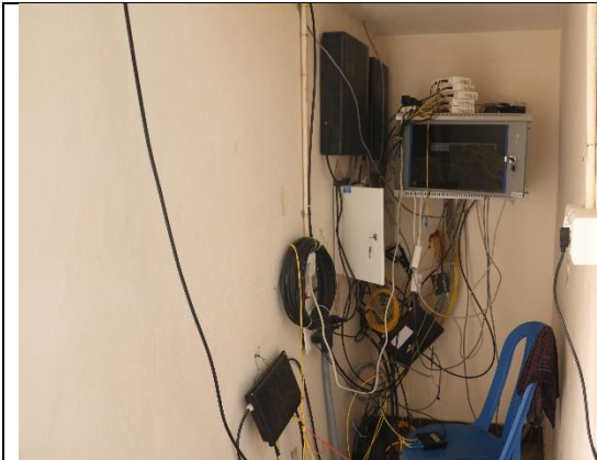
Intranet and Internet Service of Leased OFC for 20 MBPS from BSNL & Broad Band of 50 MBPS form Airtel
